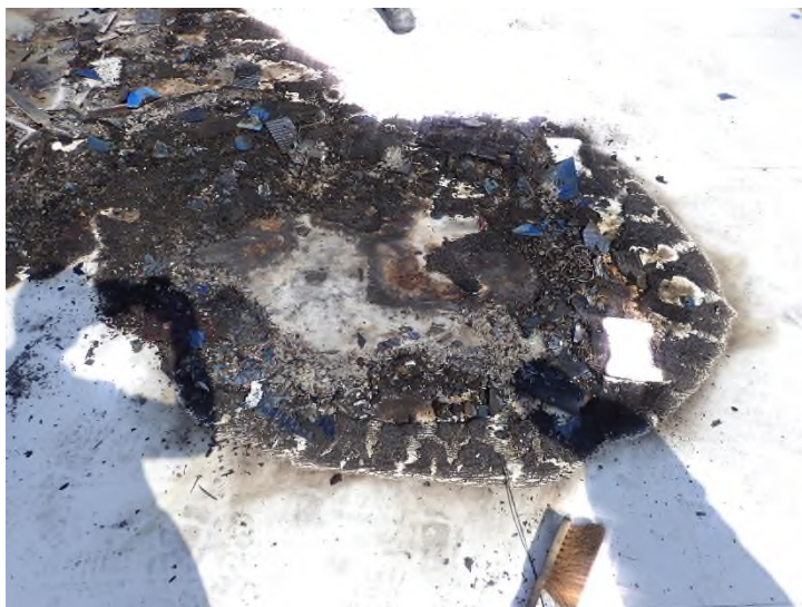
Photo 10 Overview of the burnt roof waterproofing sheet.
