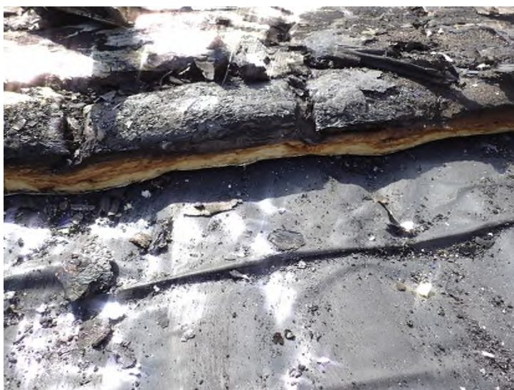
Photo 32 Overview of the burnt depth of the thermal insulation.
