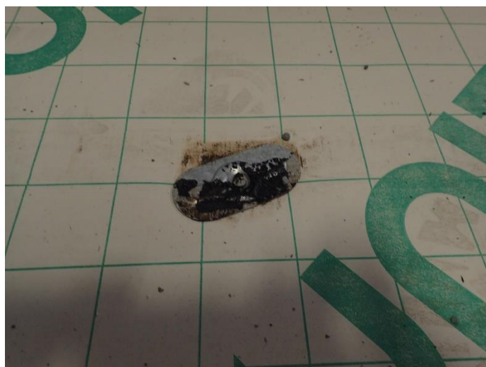
Photo 2 Detail of the failure mode.
