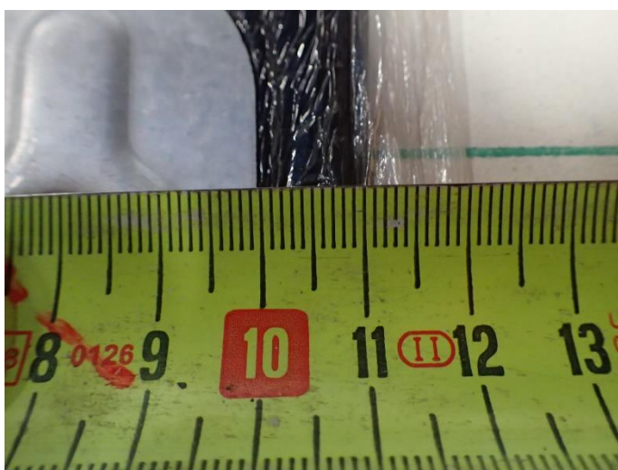
Photo 6 The distance from the edge of the fastening system to the edge of the roof waterproofing sheet.
