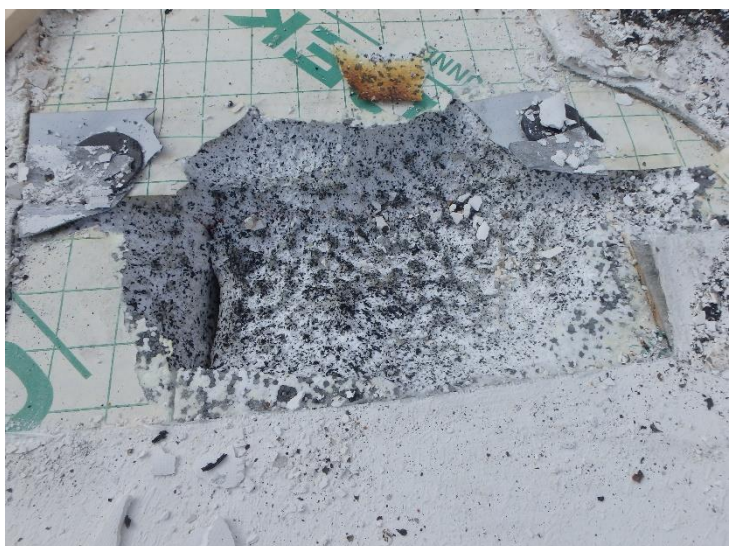
Photo 6 Overview of the damaged area of the thermal insulation.
