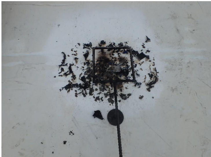
Photo 5 Overview of the damaged area of the coating.
